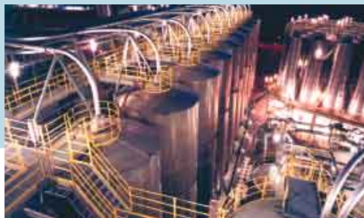
Polypropylene storage facilities at the DSM-site Geleen
